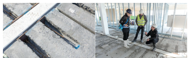
Figure 16: Floor structure photo (a) and type of connection (b) Temporary District Court
